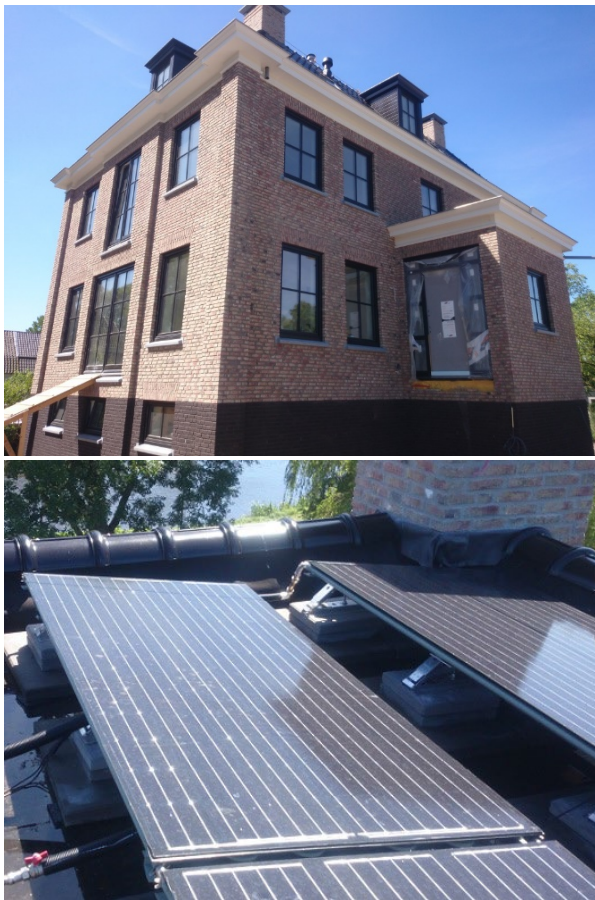
Figure 5.1. Test building near Amstelveen, the Netherlands, during the construction phase in summer 2017 (top); photovoltaic thermal solar collector (PVT) from TripleSolar on the roof of the building (bottom).
